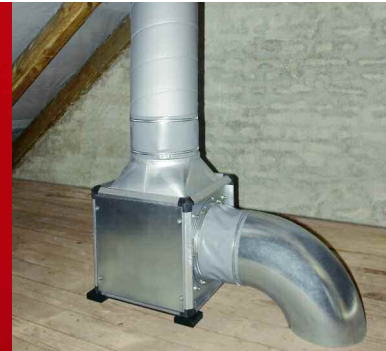
Installation in the attic with anti vibration mounts (accessories).
